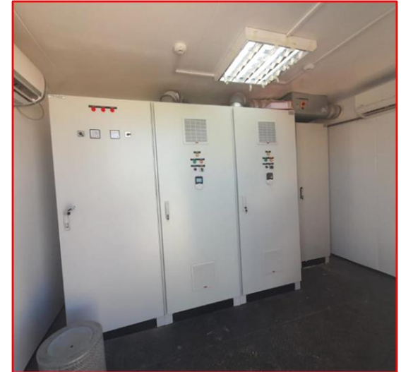
Electric station for water injection Operation
