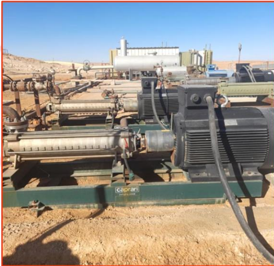
Water injection Bonassisa Operation in Tunisia – ENI site
