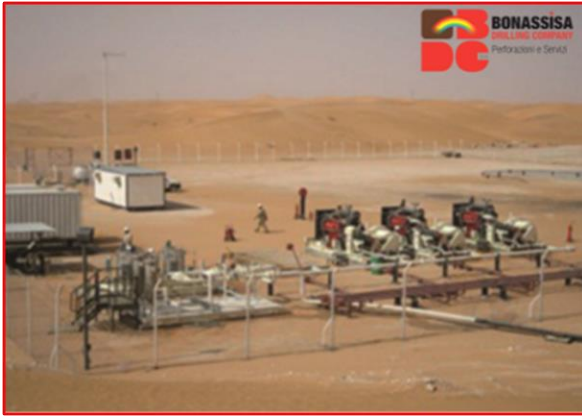
Water injection station in Tunisia – ENI site
